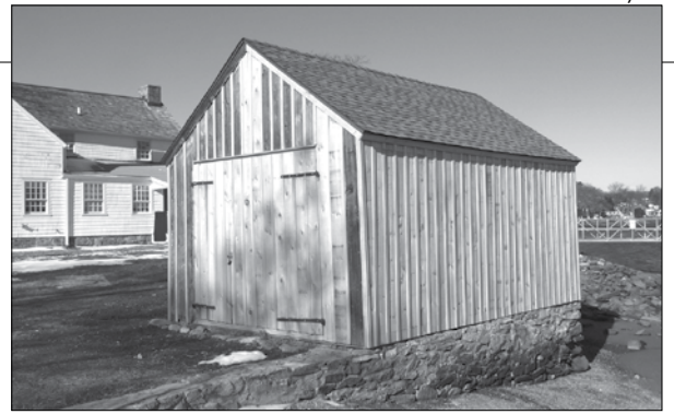
The SoundWaters shed, in Cove Island Park, Stamford, was repaired with funds from a Hurricane Sandy Disaster Relief Assistance Grant
