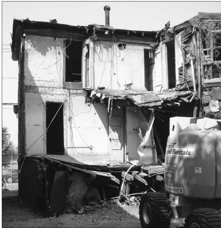
Dismantling additions on the Freeman houses, in Bridgeport, has revealed clues to the houses' history.
