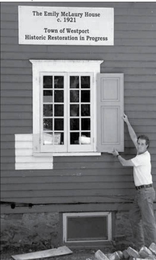
Restoration of the Emily McLaury house in Westport included repairs to historic windows and replication of the original shutters.
